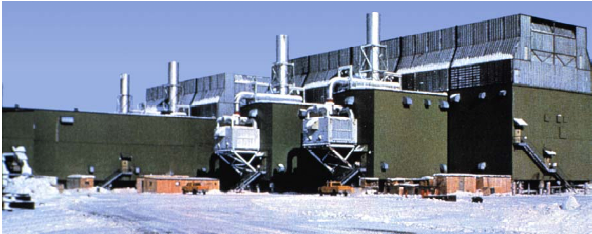
Figure 4. Winterized forced draft units
